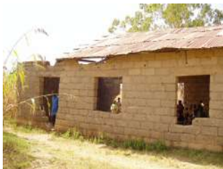
Example of Irrepairable Classroom Building (2)
