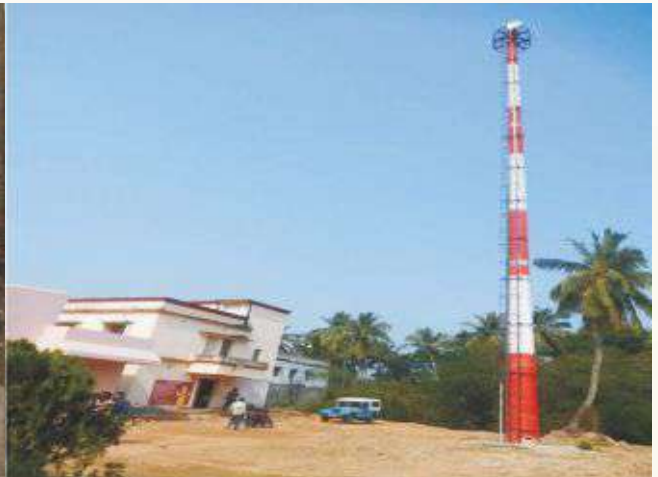
EWDS (Alert Siren) at Basudevpur, Odisha
