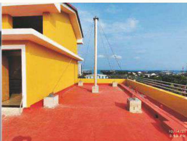
Mono pole tower of EWDS at MPCS, Goa
