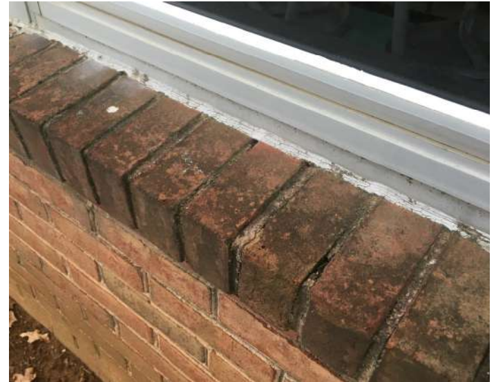
Rowlock sills in need of repointing
