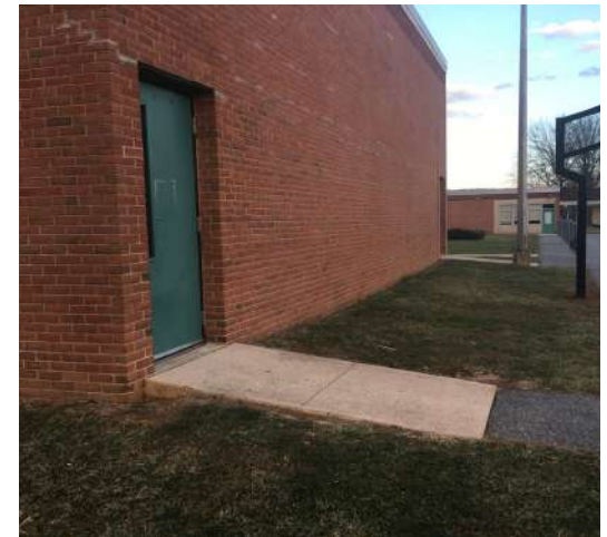
Many exterior egress doors do not have level landings at the exterior
