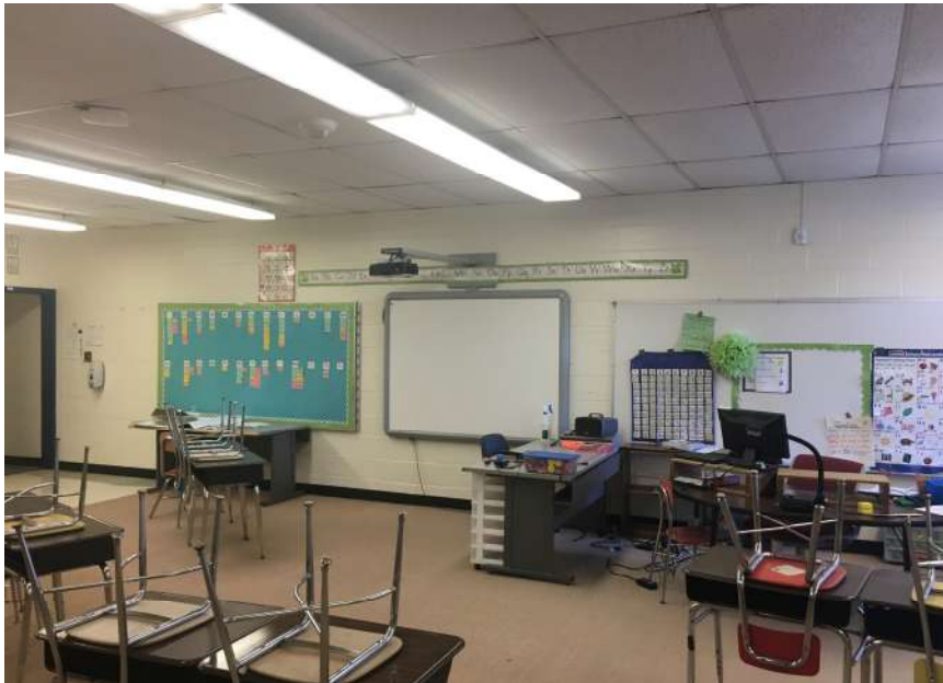
Typical surface mounted lighting at original classroom wing
