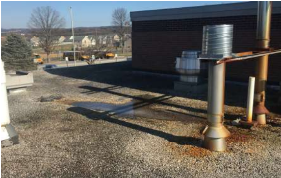
Area of standing water at mechanical room roof
