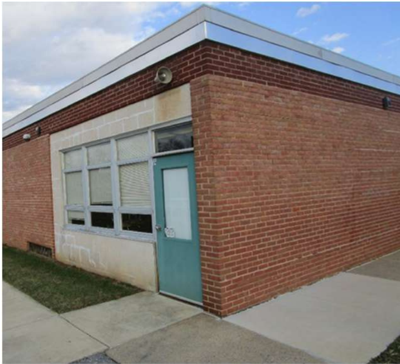
Photo 2: First Classroom Wing SW corner – possible foundation settlement
