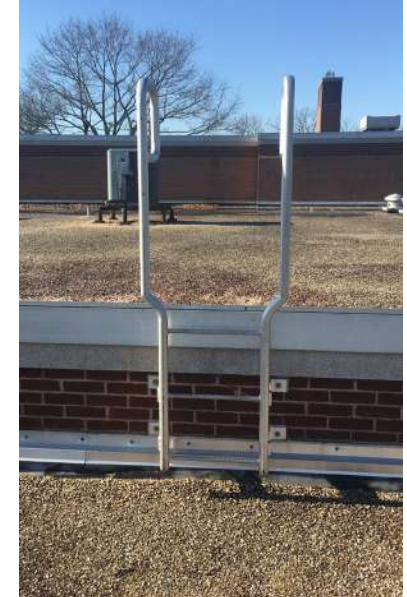
Roof transition ladder
