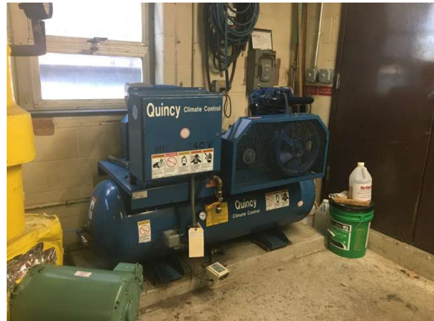
Air compressor for pneumatic controls
