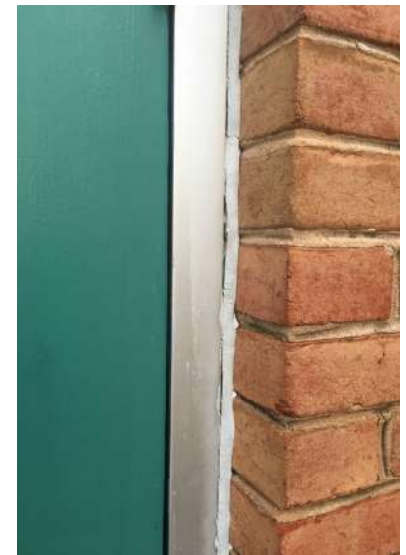
Failing sealant at frame
