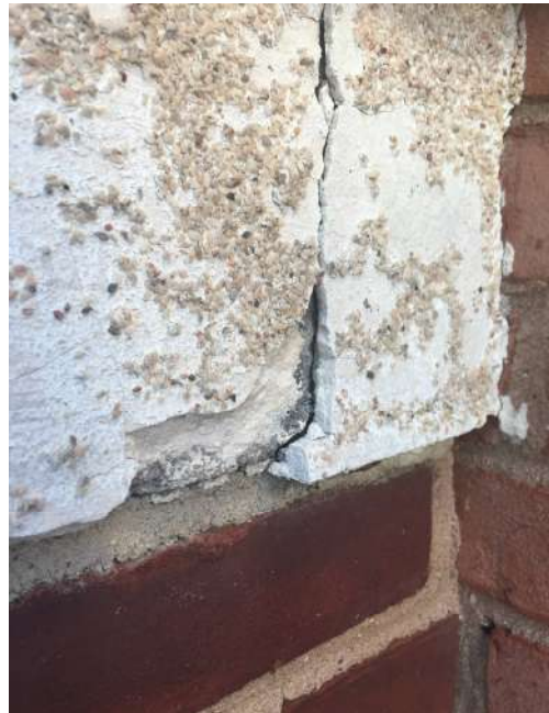
Detail of marble chip course cracking
