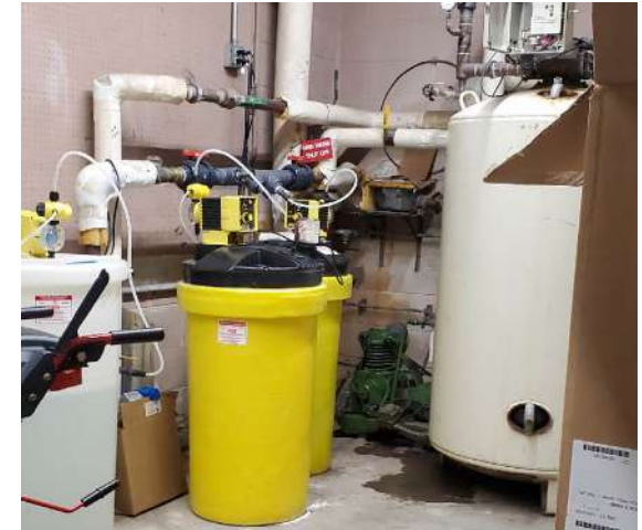
Water Treatment system
