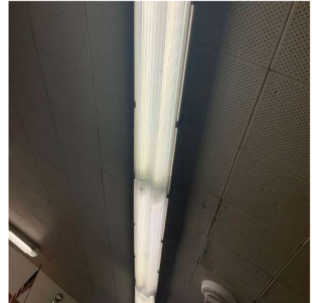
View of surface mounted lighting
