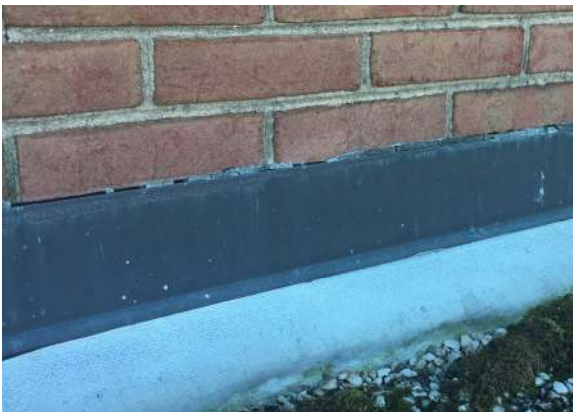
Deteriorating sealant at flashing reglet
