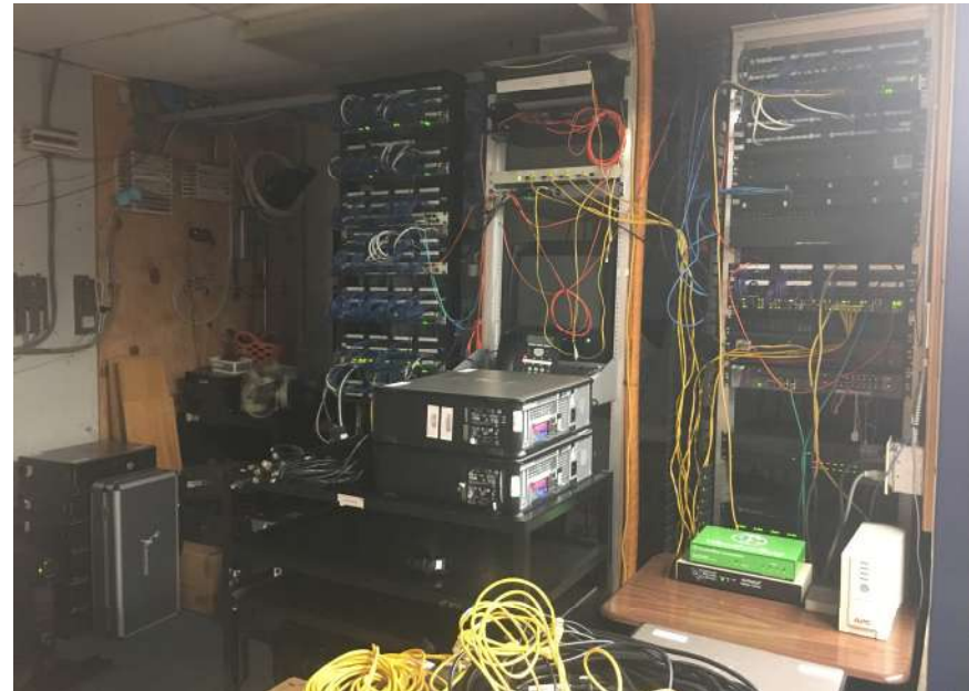
MDF closet adjacent to Media Center
