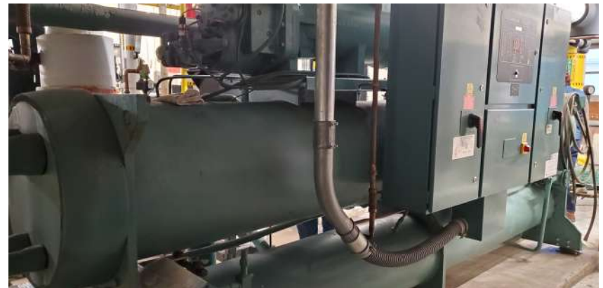
Water cooled chiller
