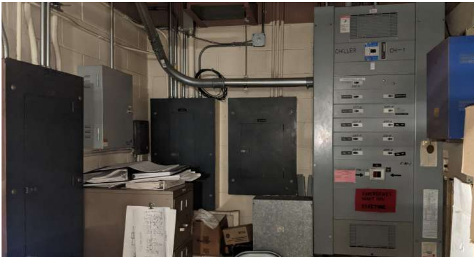
Electrical equipment and panels
