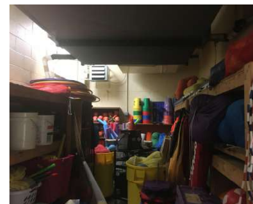
Gym unit hung in storage room
