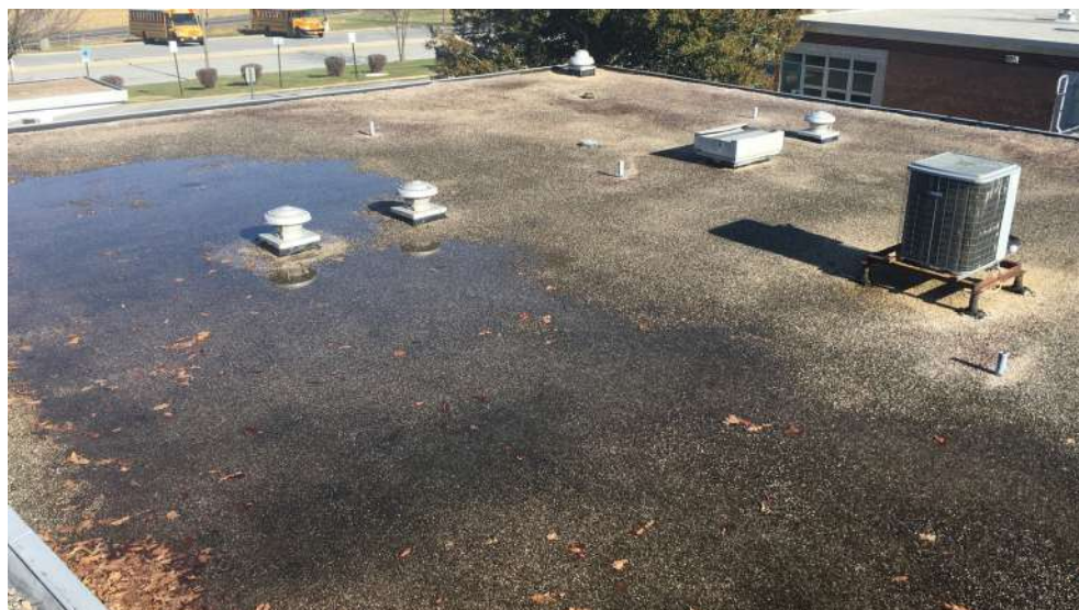
Standing water at roof area above main entry and administrative area
