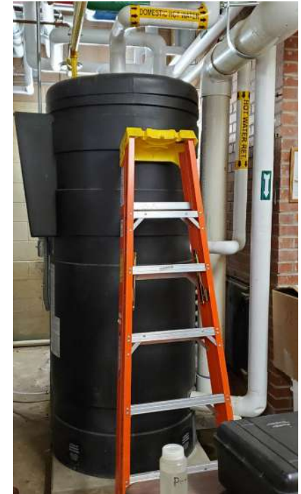
New hot water heater
