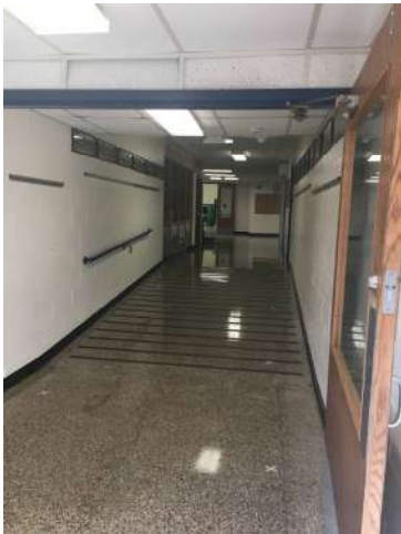
Corridor ramp is non-compliant due to slope and lack of railings
