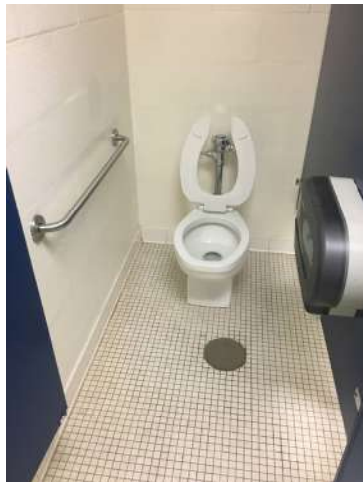
ADA stall dimensions are not met and required grab bars not provided
