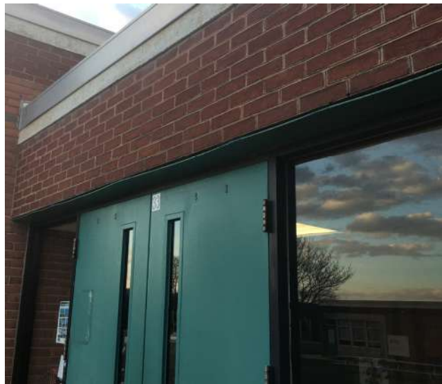
Gym addition exterior door lintel distortion
