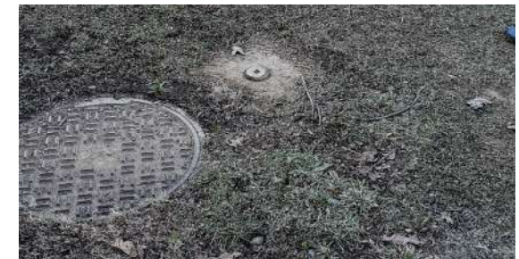
Grease Interceptor access
