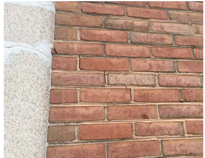
Brick corner chipped and stairstep cracking
