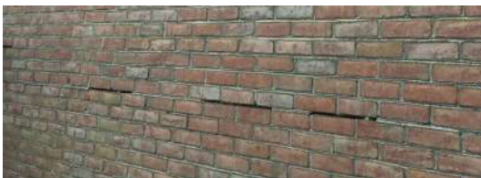
Areas of horizontal mortar joints missing
