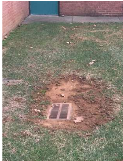
Yard inlet drainage issues
