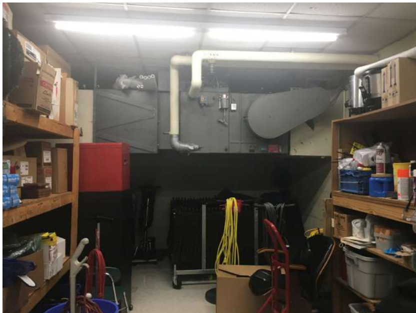
Kitchen make-up air unit hung from structure in adjacent storage room
