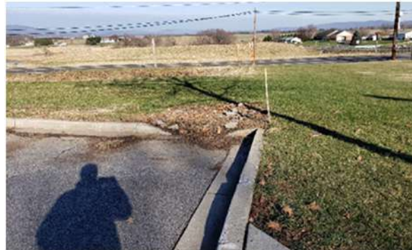
Blocked SWM inflow at north parking area
