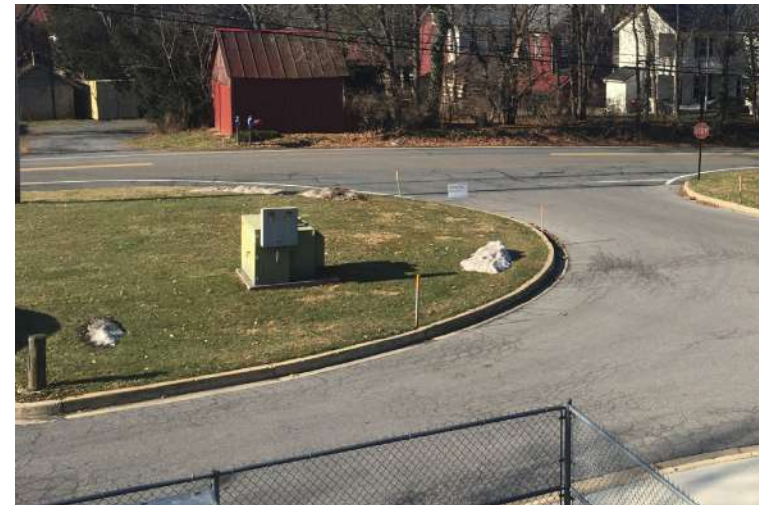
Electrical transformer near Horine Road access
