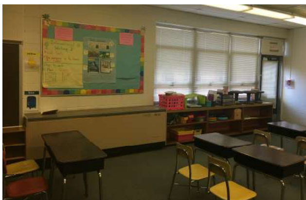
Typical Classroom unit ventilator
