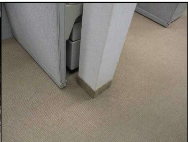
Interior column and slab obscured by carpet.
