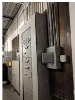
Limited electrical room serves all mechanical needs.
