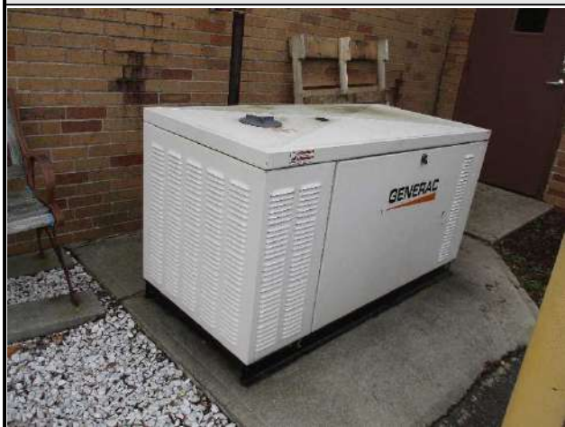
Emergency generator condition.
