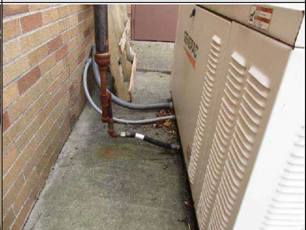
Natural gas piping to the emergency generator.
