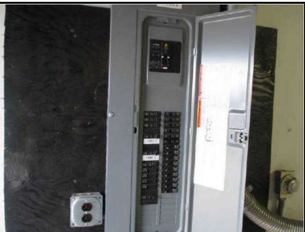
Typical electrical panel.
