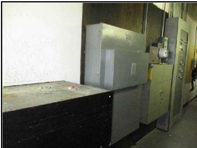
Main electrical service.
