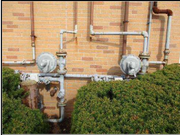
The natural gas meters located on the south side of the Subject building.
