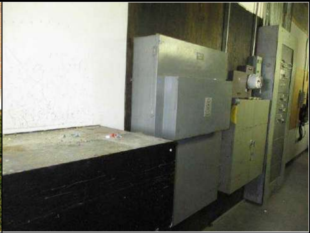
The main electrical switchgear.
