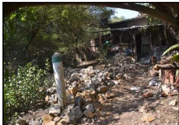
Illegal construction seen at the site
